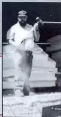
Clif Fisher of Maintenance performed a great job in some much needed renovations at the Newton Plant. Thanks Clif!
